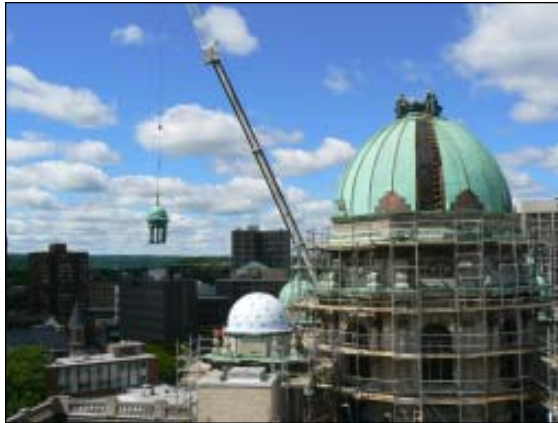
As work begins on the court house roof, the cupola is removed from the main dome.
