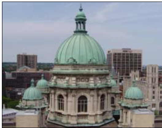
The main dome and satellite domes of the Onondaga County Court House prior to the start of roofing work.
