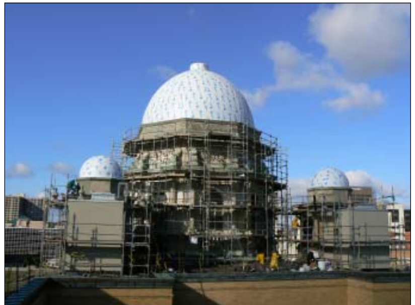
The court house domes are clad in protective self-adhering membranes until they are ready to be re-covered in new copper.
