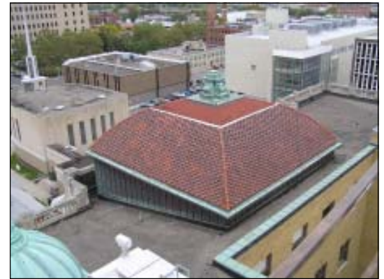
View of the north clay tile dome on the roof of the Onondaga County Court House.
